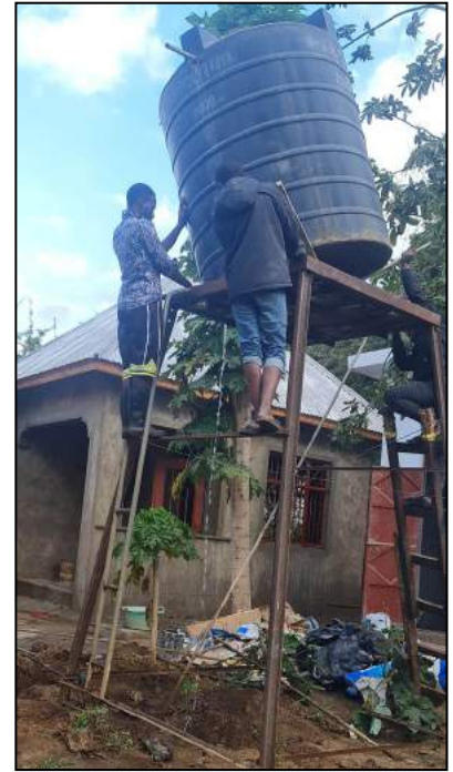
Installation of water storage tank for the house at the Mpingo Plot.
